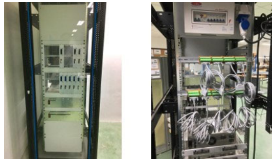
Figure 6: Equipment rack for PWM drive PCBs and DC power supply modules.
